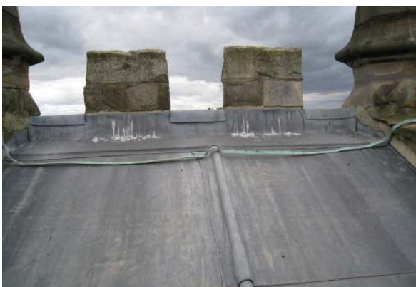
TACKED LEADWORK AND LOOSE STRAP
