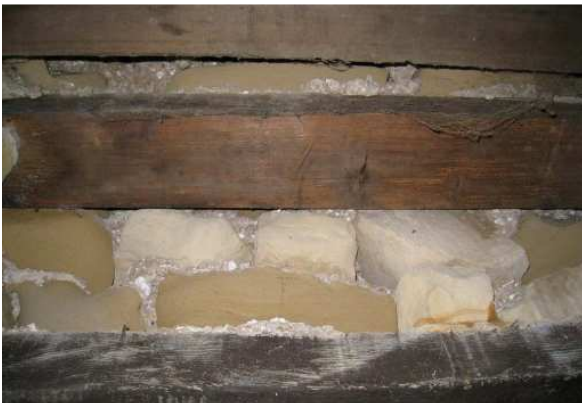
WEST GABLE EROSION
