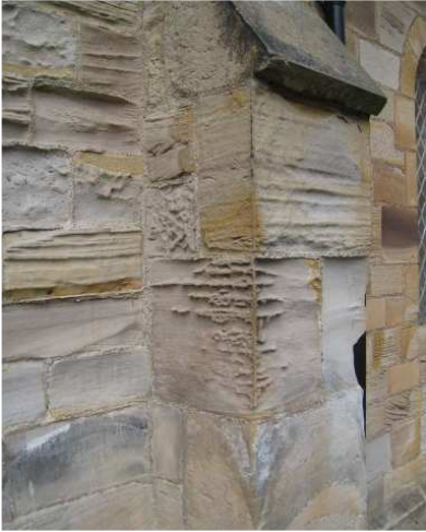
BUTTRESS BE3 EROSION
