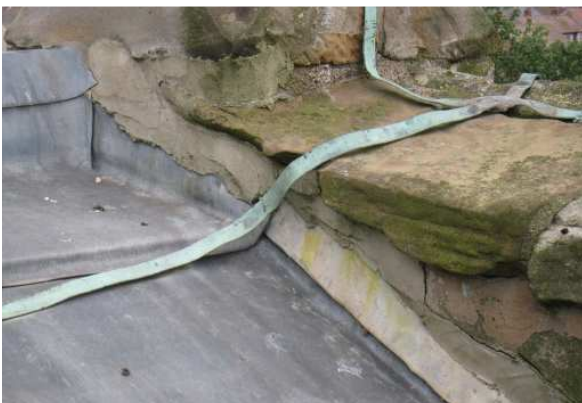
TOWER ROOF CONDUCTOR STRAP
