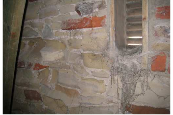
EAST GABLE STONE EROSION
