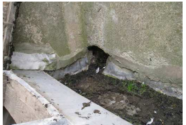
CHOKED PARAPET GUTTER
