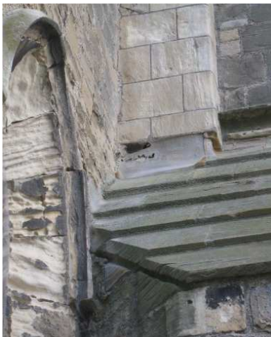
LANCET WN1 & ROOF EROSION
