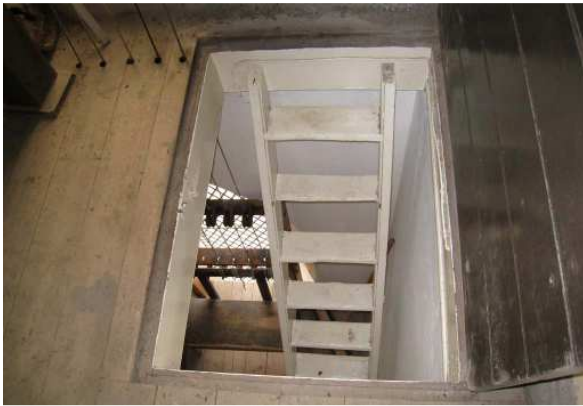
STAIR ACCESS GUARDING + GATE REQUIRED
