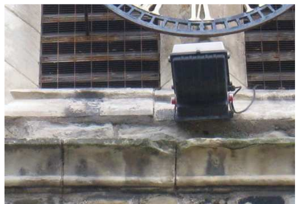
LANCET CILL OUT OF JOINT
