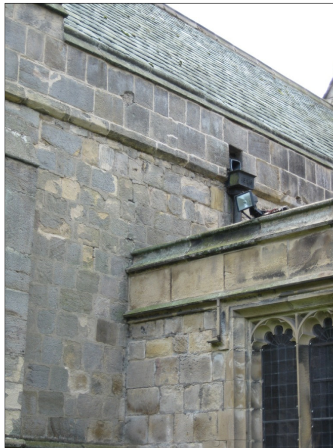
Open joints in wall of Chancel above Vestry roof
