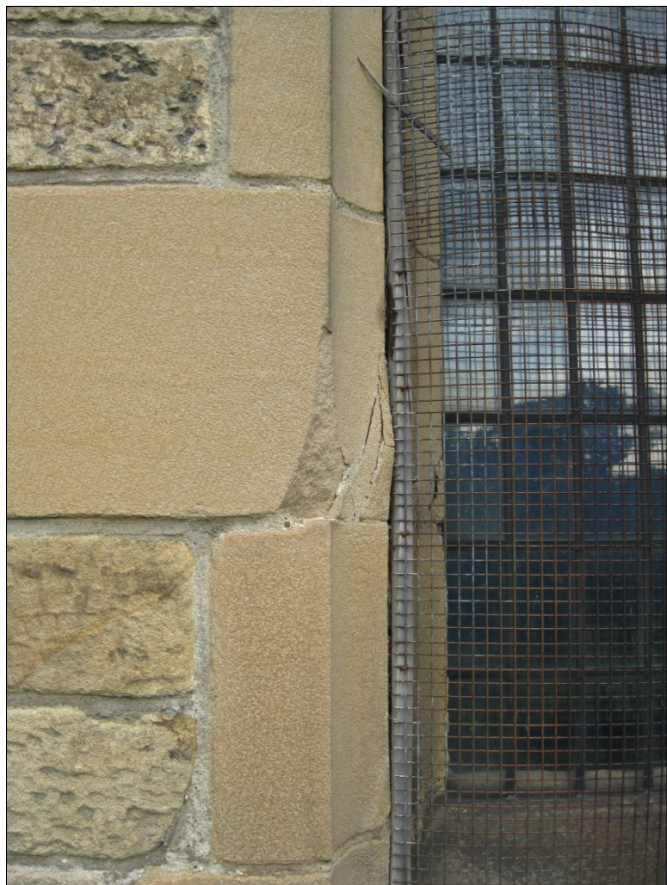
Spalled window jamb: South Aisle, West of Porch
