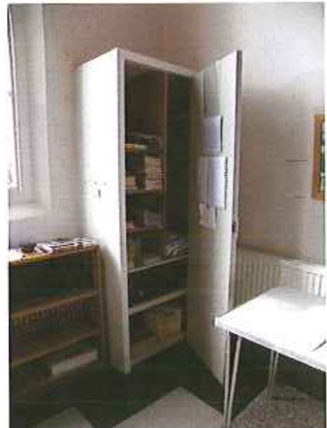
4. South West internal corner of church showing gas meter
